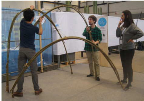
Figure 1: Setting up of the main formwork arches where the pulled fabric will then be mounted. Smart Geometry 2016. [Photo by the participants of the cluster].
